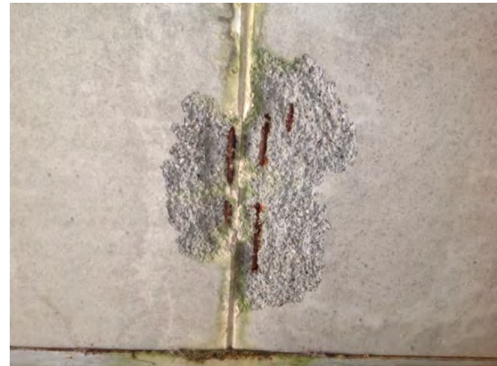
spalling concrete under panel 1 and 2 on right side
